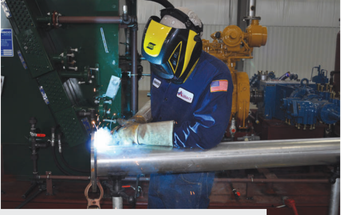
■ A welder prepares a pipe spool for a new package being fabricated in Alegacy Equipment's plant.
